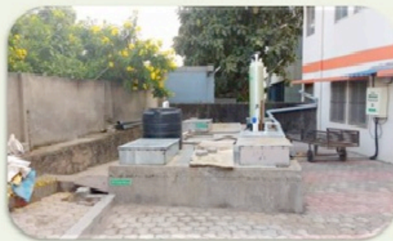
Sewage Treatment Plant (Location: Girl Hostel)
